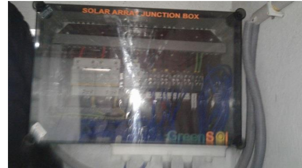
Solar Array Junction Box Cum DC DB
